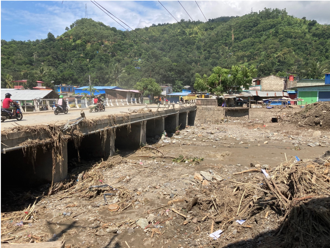
Damaged bridge by flood in Dili (photographer, Atsushi Takahashi, Project Coordinator of Project for Capacity Development for Faculty of Engineering Science and Technology, the National University of Timor-Lorosa's Phase 2 (CADEFEST Phase 2))
